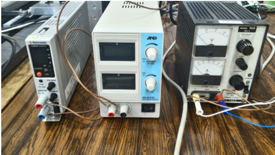
Figure 8.2.17: Power supplies for controllers
